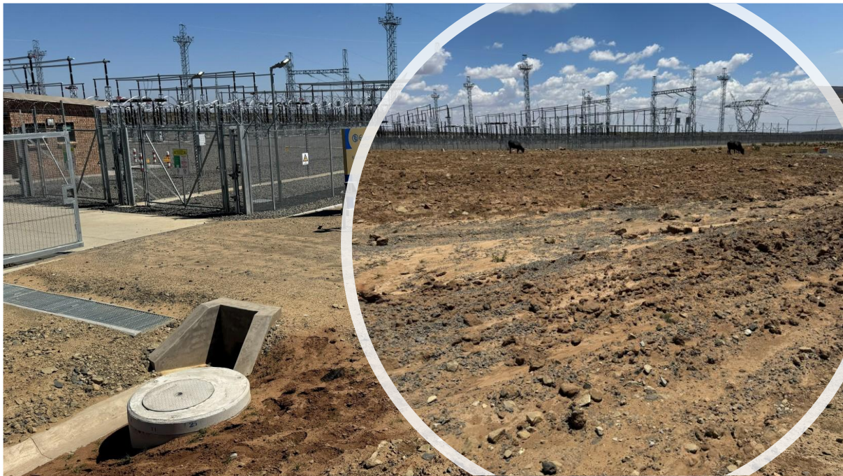
Figure 6-2: Drainage line and associated stormwater management infrastructure observed onsite.
