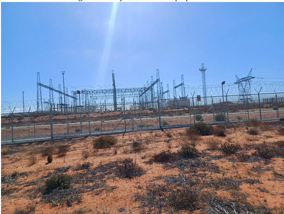
Figure 4: Existing Gromis Substation
